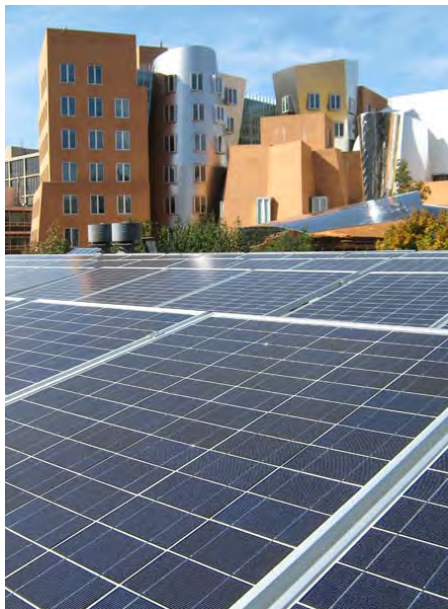
Figure 3. Photovoltaic Roof Panels
